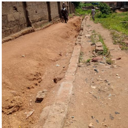
Plate C: Drainage channel completely blocked with sand
