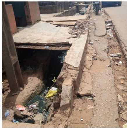
Plate B: Drainage system blocked with refuse
