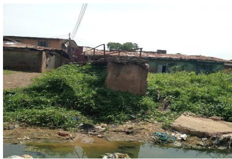
Plate A: destruction of the bridge pedestrian bridge at Kudeti
