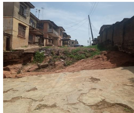
Plate B: Gully erosion almost eating up a residential house at Oke-Ado
