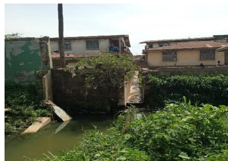
Plate B: A collapsed building as a result of erosion
