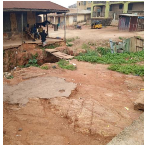
Plate D: Expansion of culvert into gully directly in front residential buildings
