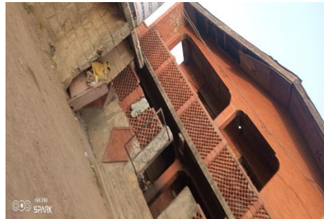
Fig. 16. Falling Ceiling Covering
