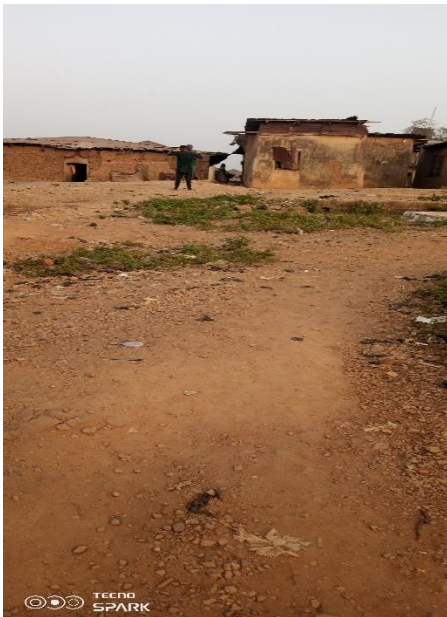
Fig 13. Exposed wall, loosed door and window
