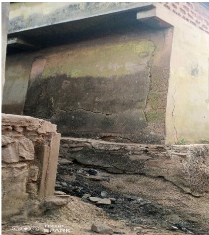
Fig. 21. Wall cracks and damp
