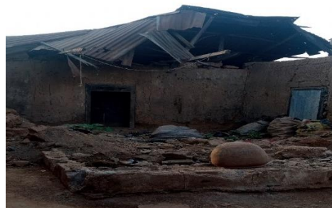
Fig.10. Twisted & Loose Doors
