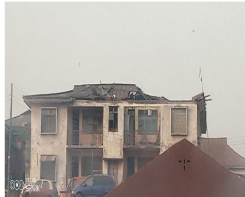
Fig 14. Open ridges, falling roof, uplifted overlaps, hanging facial, loose window and door, peeled paint.
