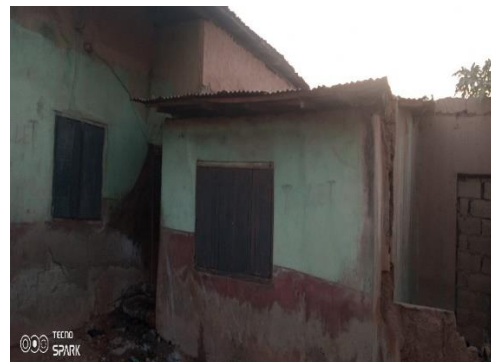
Fig. 11. Peeled paint & wall cracks
