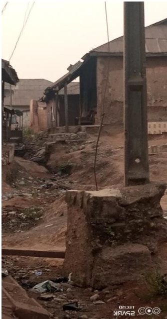
Fig. 12. Exposed foundation & rustic roof
